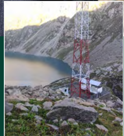
Installed BTS site at Katora Lake providing mobile coverage to the area.
